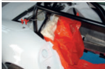
Centre: Initial seat of pipes tie wrapped to a ply base. Above: Foam finished expanding. Time to tidy up and cover the tailored seat.
